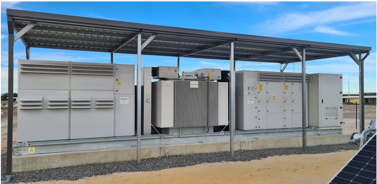
Figure 2 - Two Inverters and a Step-up Transformer (2021) https://www.fimer.com
